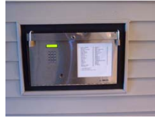
ENTERPHONE CONTROL PANEL
