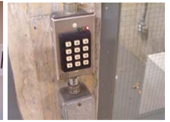
DOOR ACCESS CONTROL
