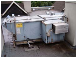
AIR MAKE-UP UNIT
