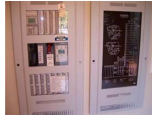
FIRE CONTROL PANEL
