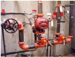
FIRE SPRINKLER VALVES
