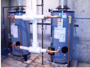
HOT WATER HEATERS
